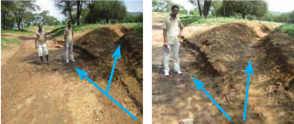
Figure 46: Imbalance in water distribution due to sedimentation at the spate flow splitting structure of Luka kebele scheme
